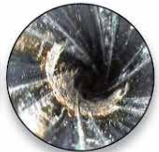
Rough patch in bore
