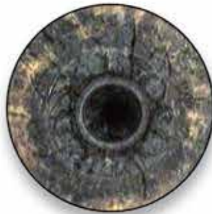
Erosion in chamber
